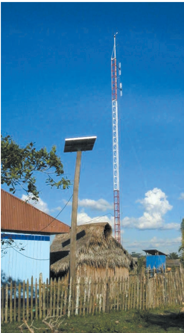
Fig. 1. Server and battery loader at the health center (HC) of Shucushyacu.
