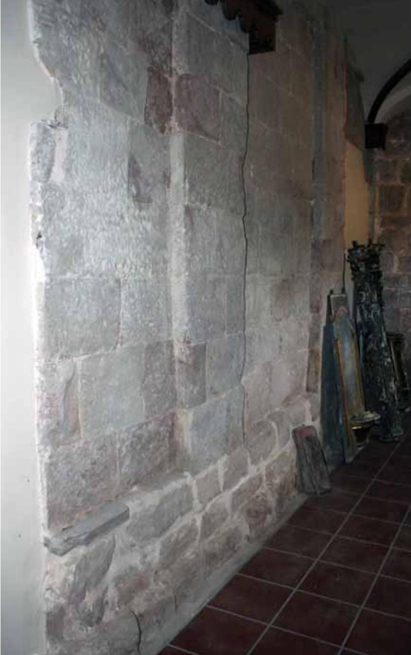
ILLUSTRATION 15. SANTA MARÍA DE VILLAVELAYO: BLIND ARCHES THAT RUN ALONG THE NORTH WALL (PHOTO: FÉLIX PALOMERO).
