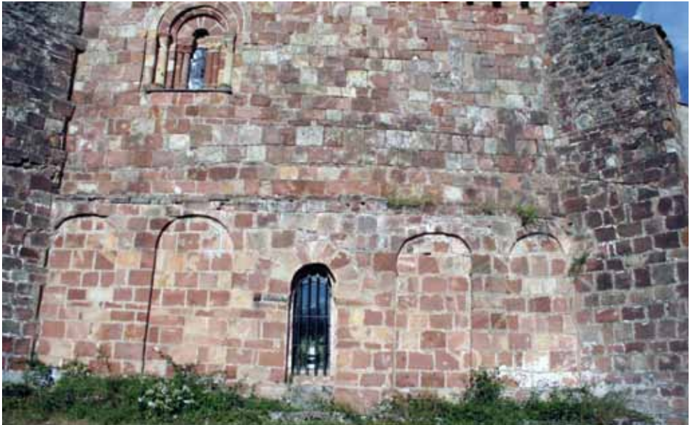
ILLUSTRATION 13. SANTA MARÍA DE VILLAVELAYO: BLIND ARCHES THAT RUN ALONG THE WEST WALL (PHOTO: FÉLIX PALOMERO).
